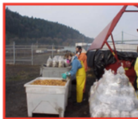
Project Setup – Sediment is contaminated with benzene, toluene, ethylbenzene, and xylene (BTEX), PAHs, phenols, and cyanide
